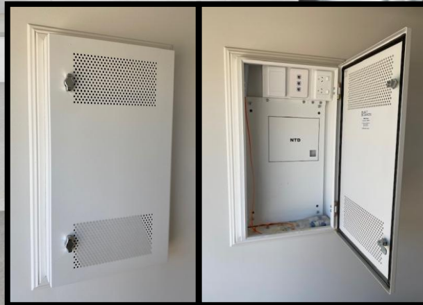
NBN COMMS BOX
